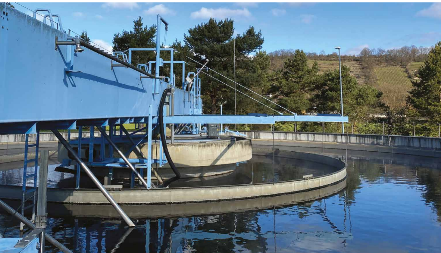
Treatment plant of Papierfabrik Palm in Eltmann.
